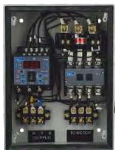
Interior View of MD Starter+ DOL Starter
