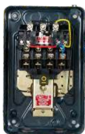
Interior View of MK1 DOL
