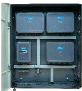
Interior View of xMasm10 - Wired Solution
