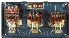
Interior View of MK2 SASD
